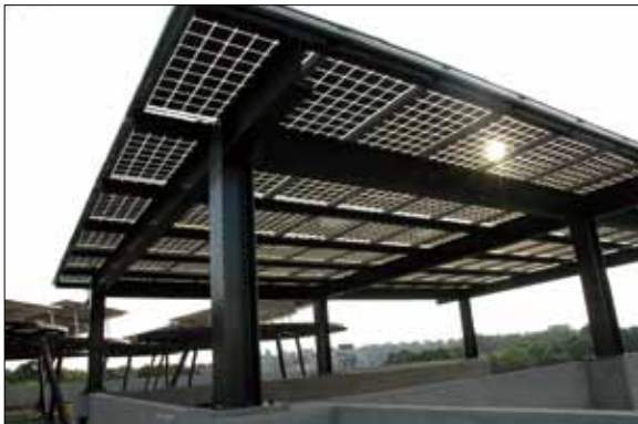
↑ Solar panels installed on roof of plant.
